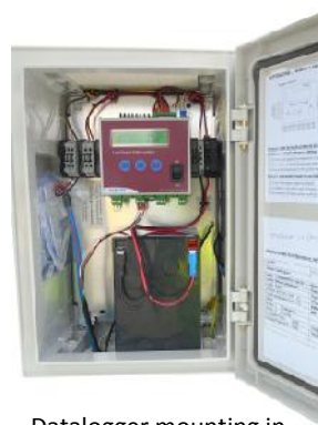
Datalogger mounting in the IP65 container
